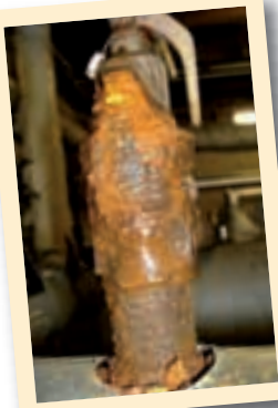
Above: corroded and scaled plant safety valve
